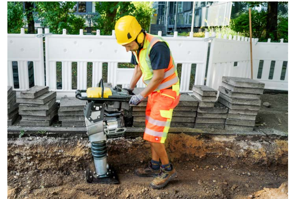
The Munich-based construction company Nibler put zero emission light equipment, excavators and wheel loaders to the test and was impressed with the results.
